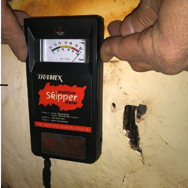
High moisture in way of loose fibreglass
